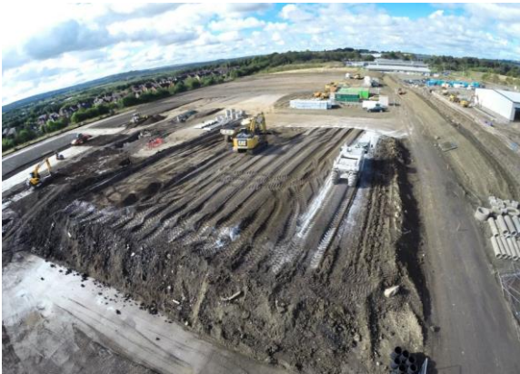
Figure 1. Lime modification for upfilling of construction podium (courtesy of Ground Developments Ltd)
